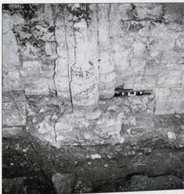
Plate 14. RA 1973: E end Chapels. The central pier between the openings through the retro-choir wall viewed from the E. The post-Dissolution blocking of the retro-choir wall is clearly visible to right (1009) and left (1039) of the picture. (Photograph Kevin Stubbs/TVAT)
