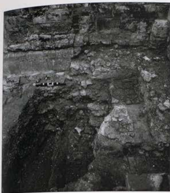
Plate 11. RA 1973: NW corner of the east end chapels viewed from the E. The post-Dissolution blocking (1009) of the retro-choir wall is clearly visible to left of the picture. The remains of the respond (context 1003) in the NW corner are visible. (Photograph Kevin Stubbs/TVAT)
