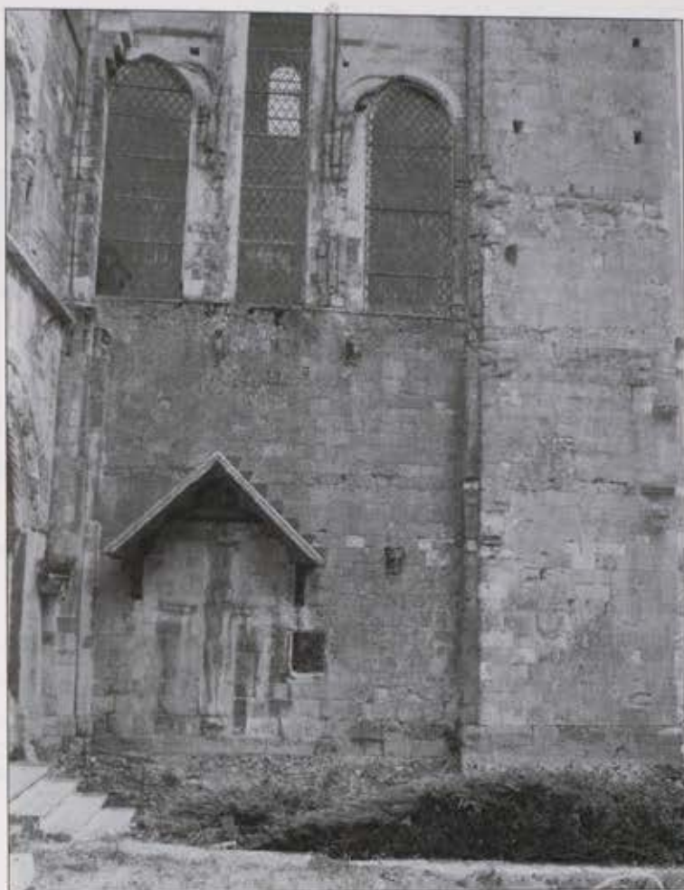
Plate 9. The W side of the S transept, showing two sets of corbels set into the wall. Note the position of the large rood. (Photograph TVAT)
