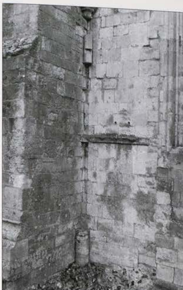
Plate 12. Detail of the respond (RA 1973, context 1037) in the SW corner of the chapel viewed from the NE. (Photograph TVAT)
